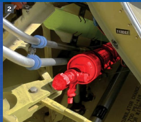
Figure 1: Installed location of the accumulator in the aircraft
